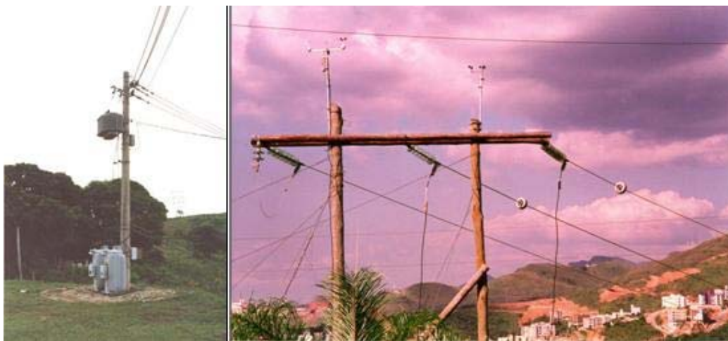
Figure 2 – Power Transformer System (300 kVA), two Reguladores de Tensão, Power Donut Sensor of Monitoring Temperature System and Weather Station in Experimental Line
