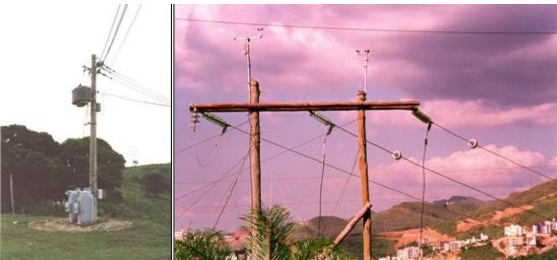
Figure 2 – Power Transformer System (300 kVA), two Reguladores de Tensão, Power Donut Sensor of Monitoring Temperature System and Weather Station in Experimental Line
